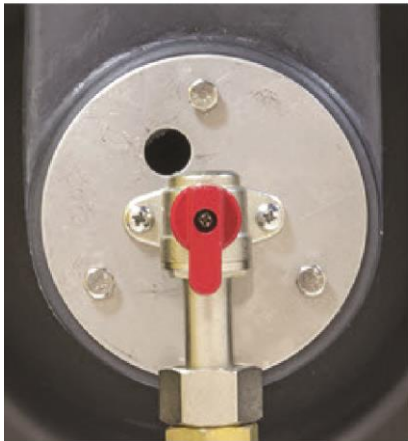
Shut-off valve OPEN
